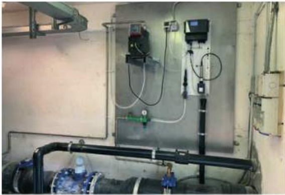
Photo 4 Acidification plant in the pumping station.
